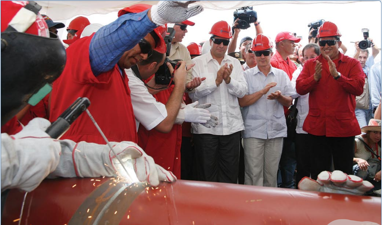
The presidents of Venezuela, Colombia and Panama attended the ceremony marking the start of the TransCaribbean Gas Pipeline's construction. Here they witness the first welding operation of this integration project.
